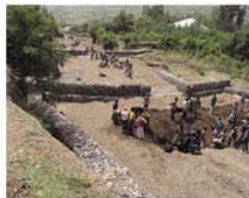
Gabion Check Dams & Retaining Walls Constructed at Kundi Sedeka Micro Watershed Site
